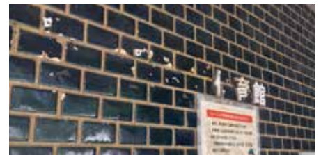
The exterior of the Training Gym. The dilapidated sign, formerly reading 'トレーニング体育館', now only reads 'イ育館'. Photo by author.
